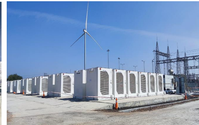
BESS, Peak Power, Karnataka
